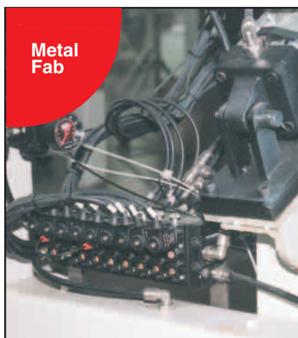
Module/Air 2000 Regulator and Stacking ALPHA Valves control Provenair Cylinders in a metal fab shop
